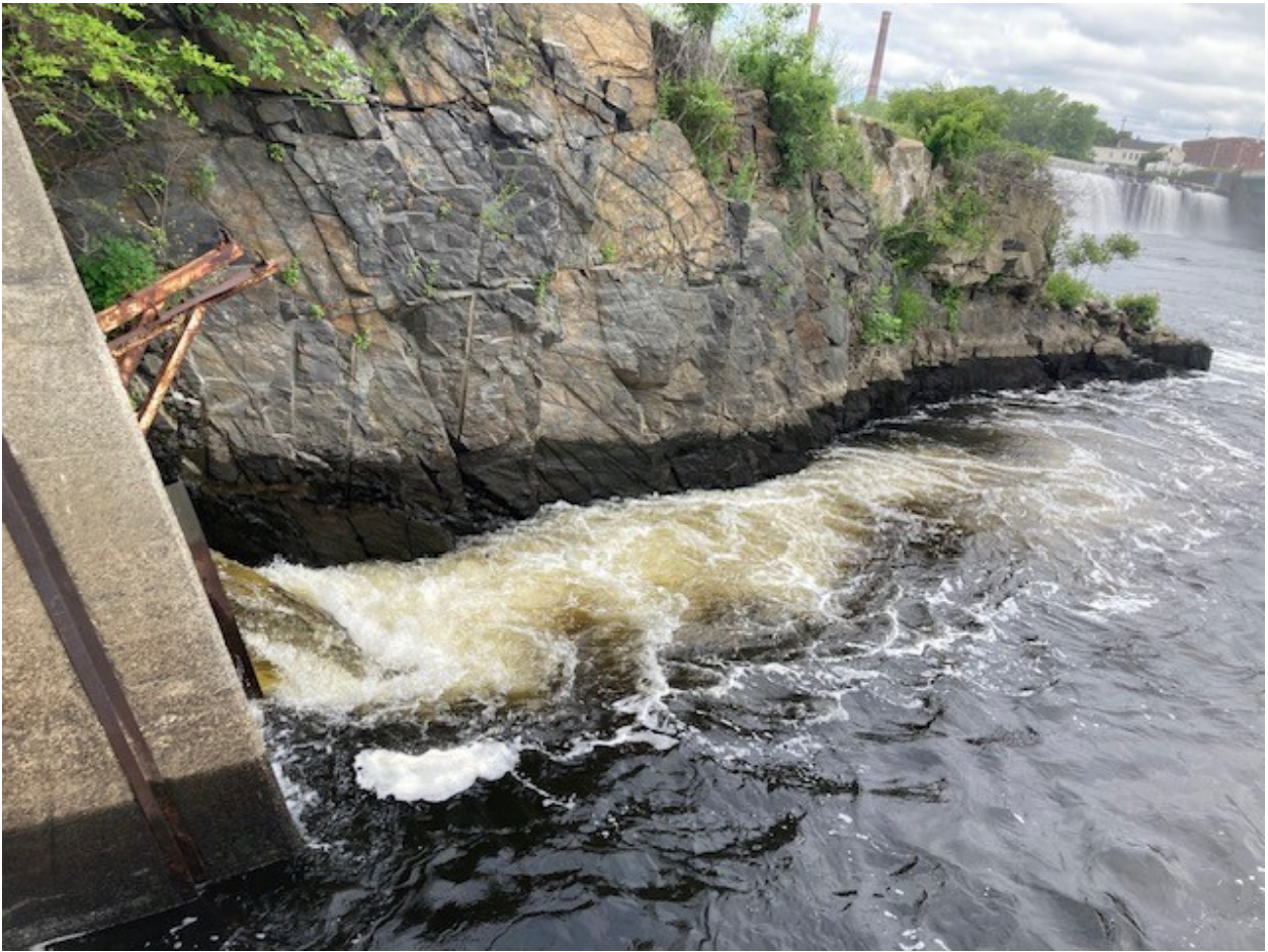
Figure 6: Perched fishway entrance conditions as water levels dropped suddenly in the tailrace.
